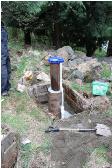
Photograph 3: The area around the well casing was excavated and a form was placed around the casing. Bentonite was placed in the excavation and the form and hydrated to establish a seal around the well casing. The well was secured with a lockable cap.
