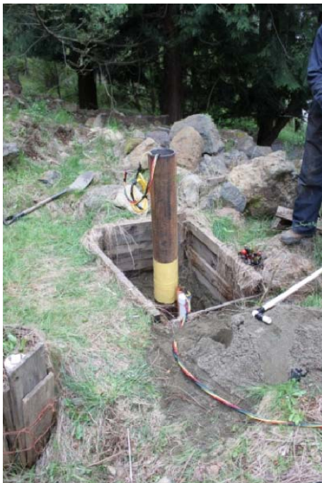
Photograph 2: The well casing was extended so that the top of casing would be greater than 0.3 m above ground surface adjacent to the well following removal of the retaining walls and regrading of the area.
