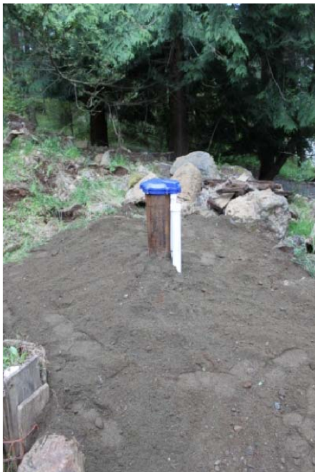
Photograph 4: The wooden retaining walls were removed and the well pit was filled with clean fill materials. Ground surface was graded to convey surface water away from the wellhead. A well identification plate was attached to the well casing.
