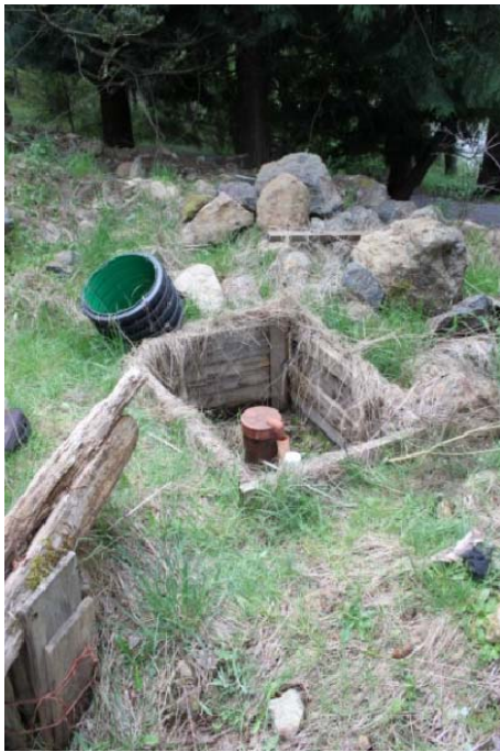
Photograph 1: Pre-existing condition of monitoring well DOH-04A. The well was completed in a well pit and the casing did not extend a minimum of 0.3 m above the floor of the pit, as required under the BC Ground Water Protection Regulation.
