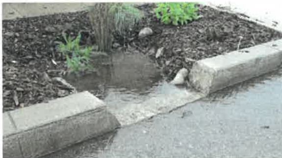
Curb cuts direct stormwater from street to landscape areas.
