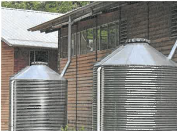
Cisterns can store rainwater to be re-used for future landscape irrigation.
