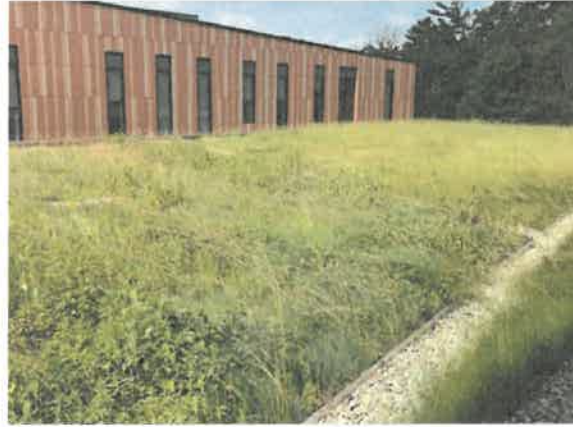
Green roofs provide shade, remove heat from the air, and reduce temperatures of the roof surface and surrounding air.
